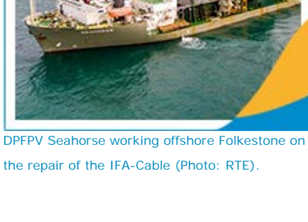
DFPPVV Seahorse working offshore Folkestone on the repair of the IFA-Cable (Photo: RTE).
